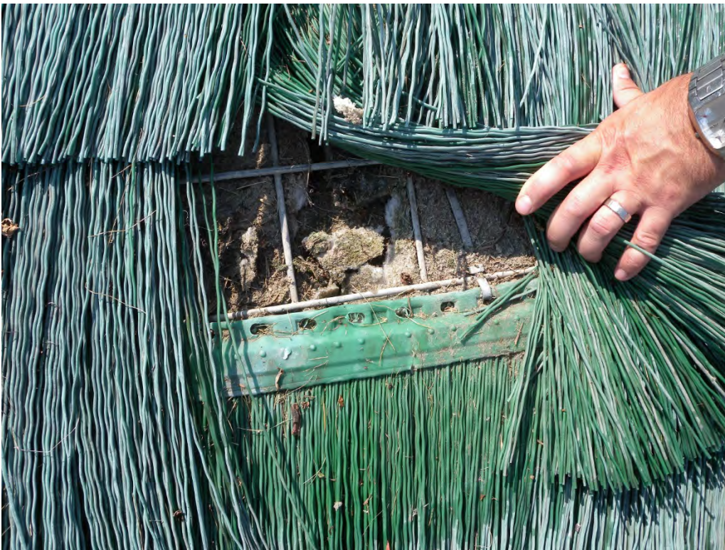
no safety plates and rotten foam mat under grating
