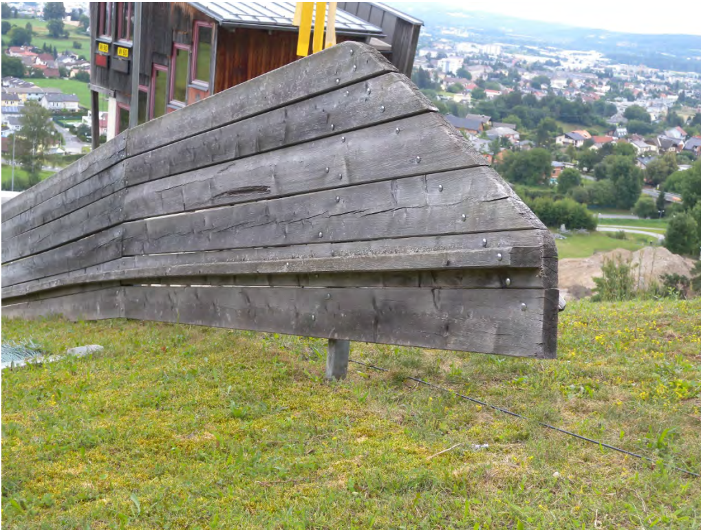
slots because of sunken ground
