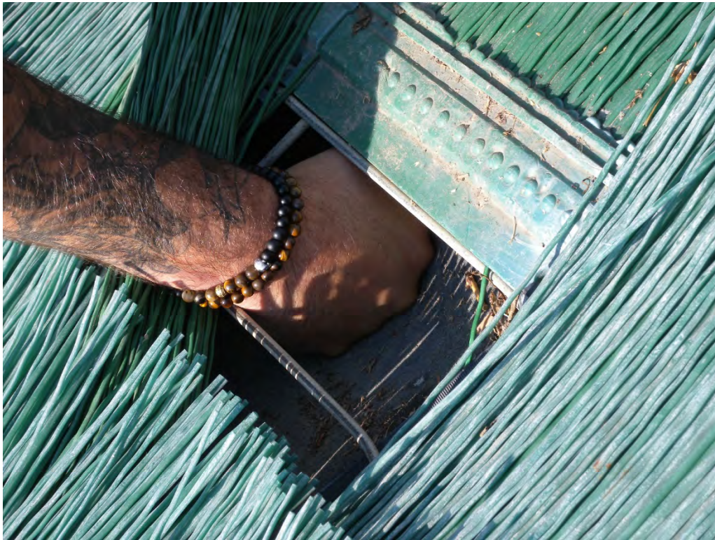
erosion of material / settling of material underneath mat cover
