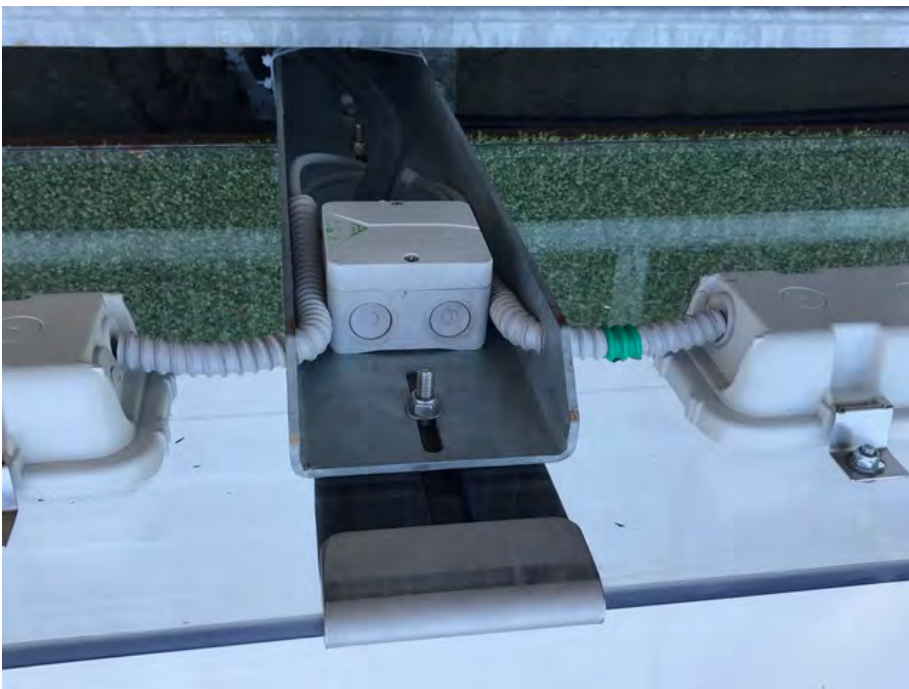
electrical installation mounted outside of sideboards - OK
