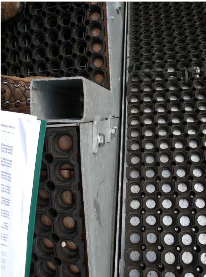
protruding screw heads
