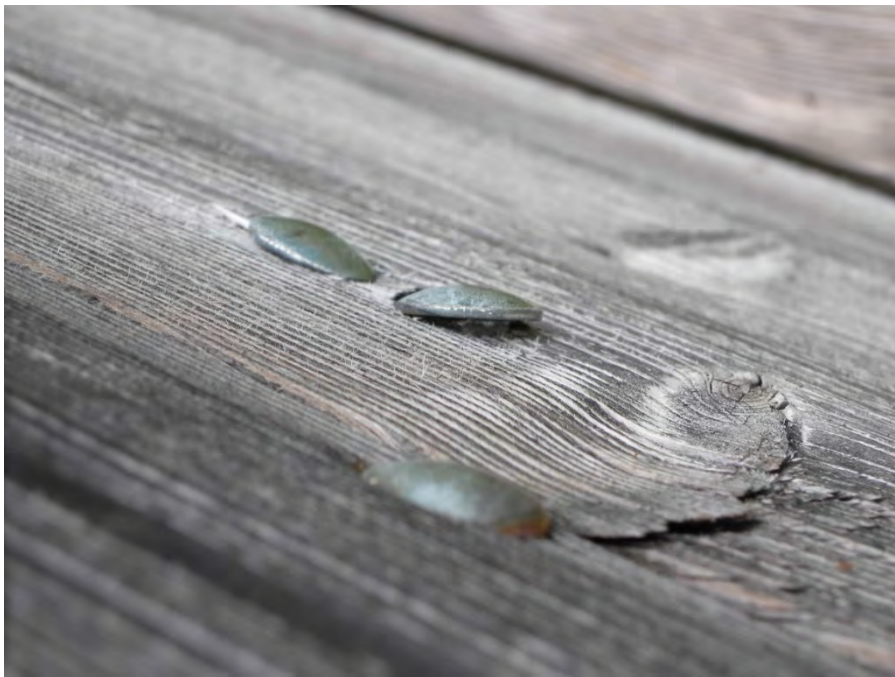
protruding screw heads – round head OK, but it has been inclined because of moving of timber
