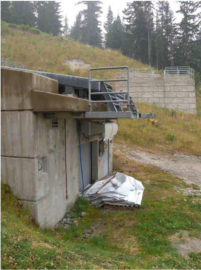
bumping mat under table and covering of steel construction with soft mat necessary
